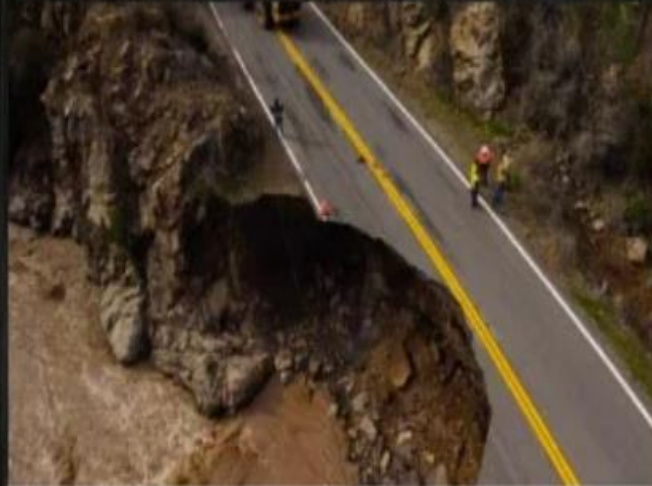
Mudslides and Road Erosion
